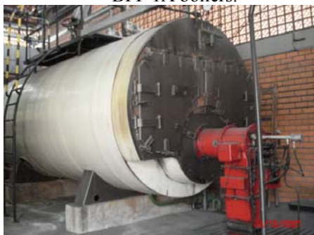
Figure 5b – One of three residual fuel oil BPF 1A boilers.
