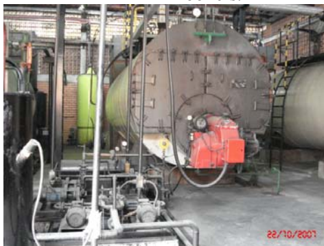
Figure 6c – One of three residual fuel oil BPF 1A boilers.
