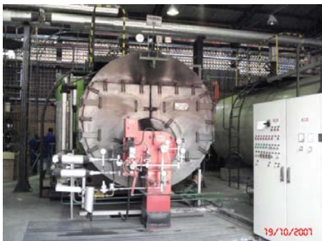
Figure 4a– One of three residual fuel oil BPF 1A boilers.
