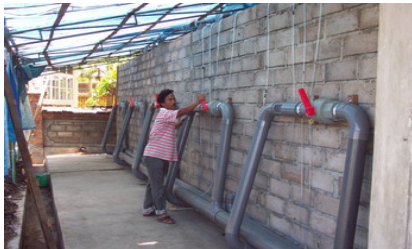
Control of laminar flow boxes
