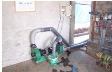
Blowers and flow controls
