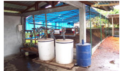
Drums for laminar research with pressure and vacuum, which is preferred by the project
