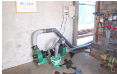
Blowers and flow controls
