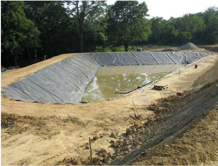
The leakage water tank.
