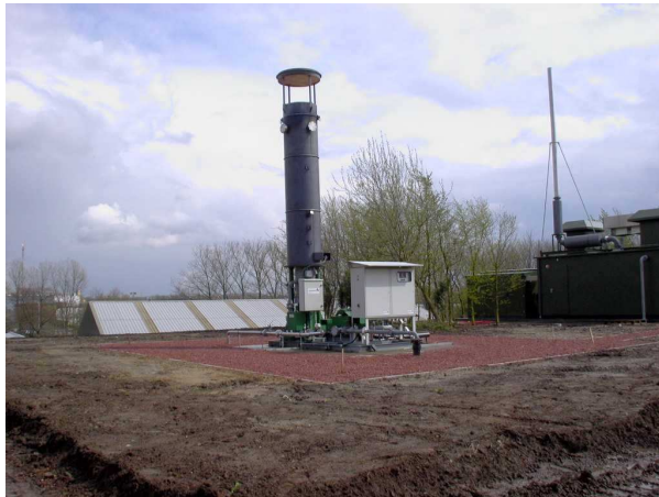
Typical biogas extraction unit
