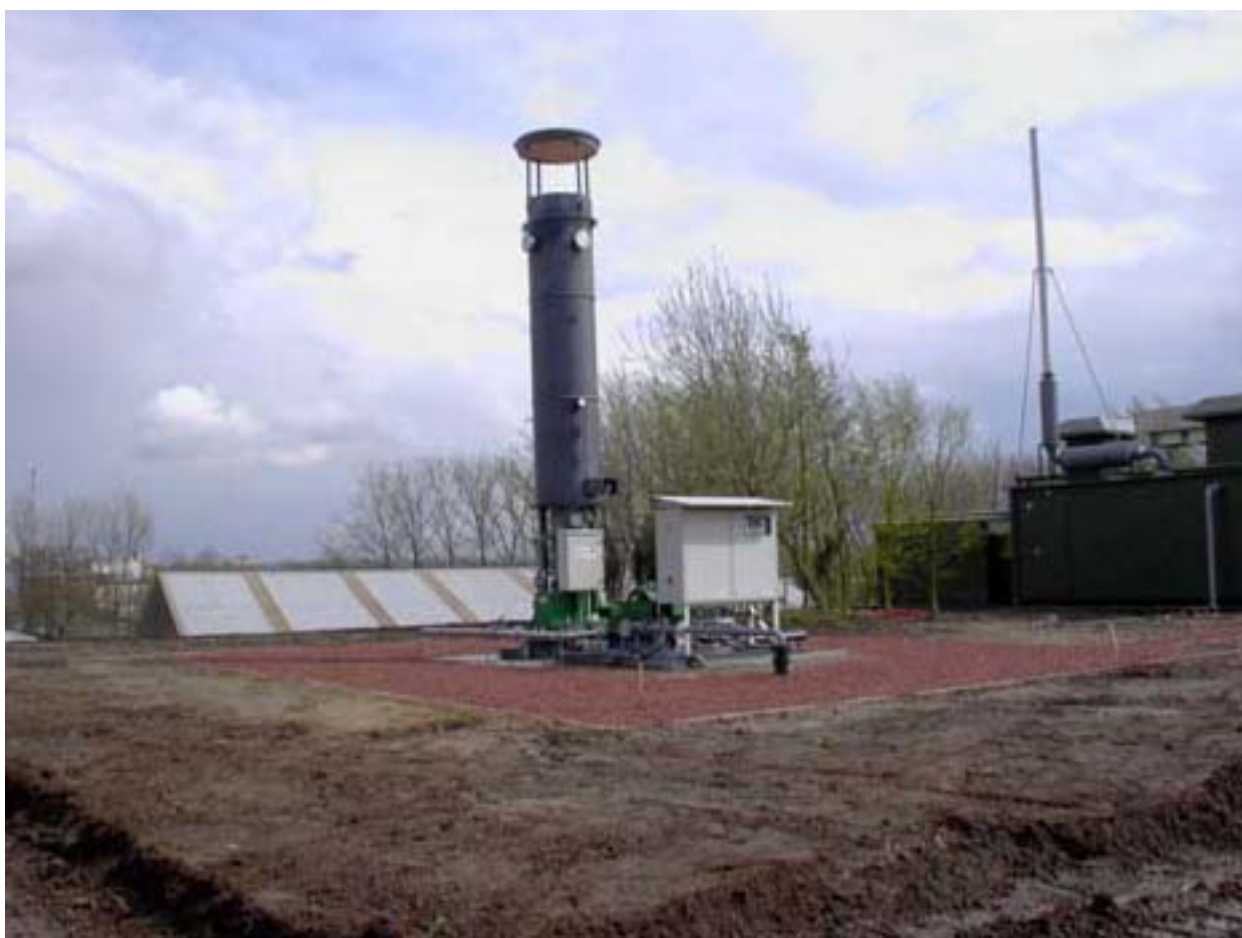
Typical biogas extraction unit
