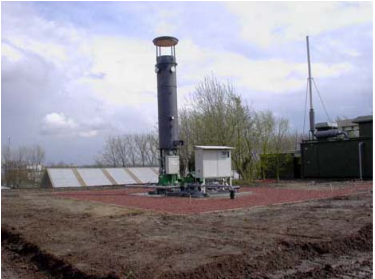
Typical biogas extraction unit.
