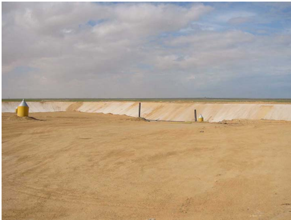
Figure 2 : Vent system in cell 2 of El Hammam landfill
