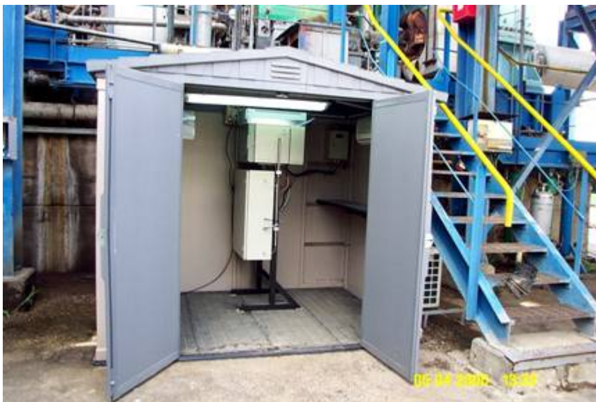
AMS Equipment inside analyzer house:
